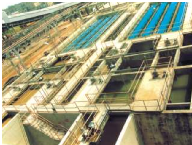
Installation of 19 MGD inclined plate clarifier at a 2 x 250 MW thermal power station.
